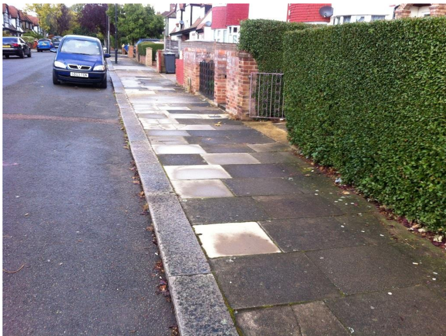
Medway Gardens - Original dark coloured slab paving is still exists, with lighter newer slabs being evidence of where repairs have had to be carried out
