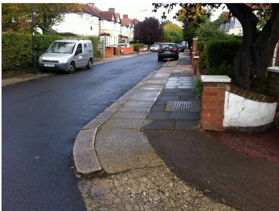
Medway Gardens: significant deterioration of concrete verges and crossovers can be seen
